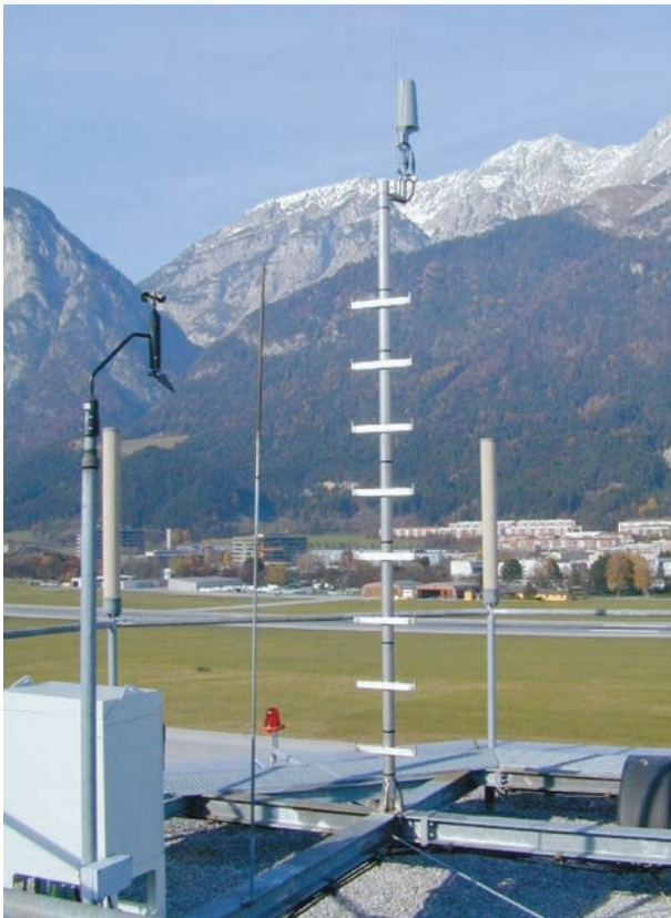
Sensor Installed at Innsbruck Valley
